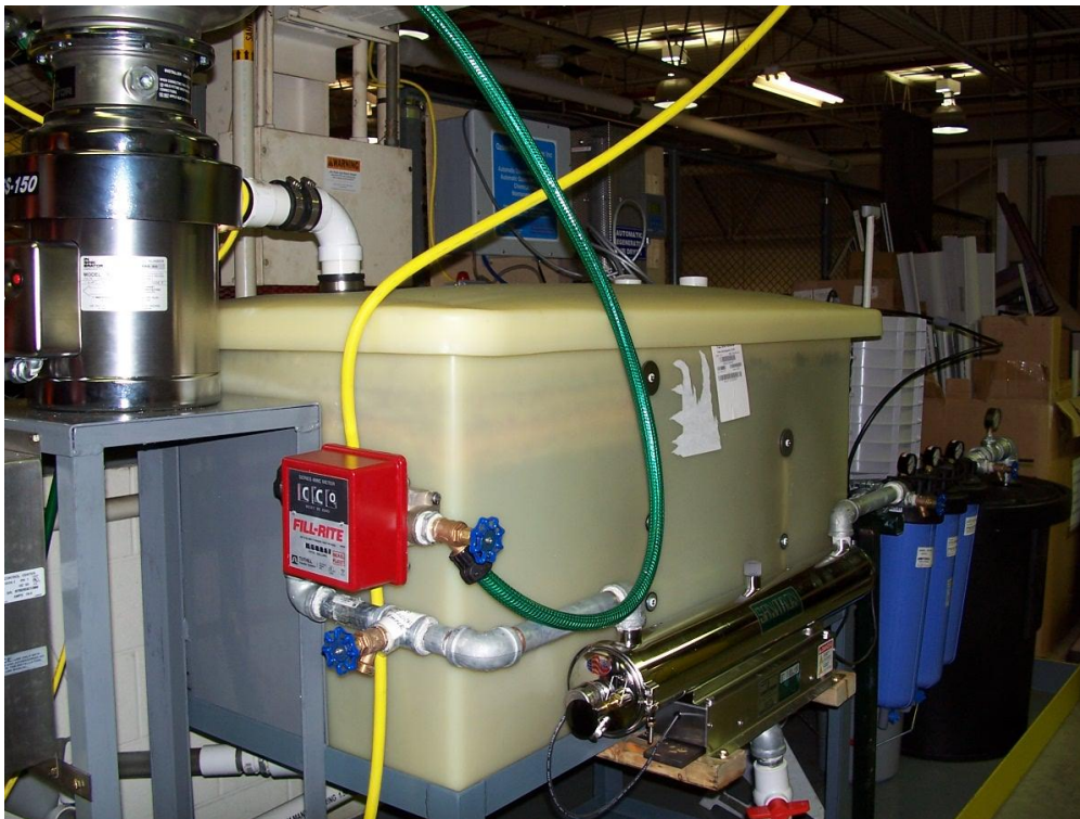
LAB SCALE SLURRY SYSTEM AT INSINKERATOR IN RACINE, WI
