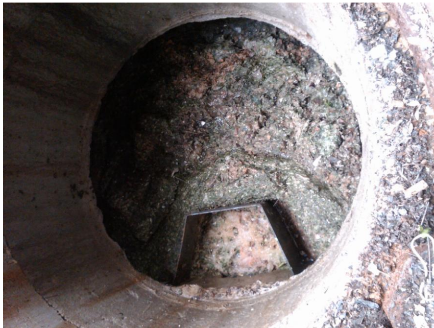
SLURRY TANK MANHOLE WITH SOLIDS BUILDUP CONCENTRATING NEAR THE INLET
